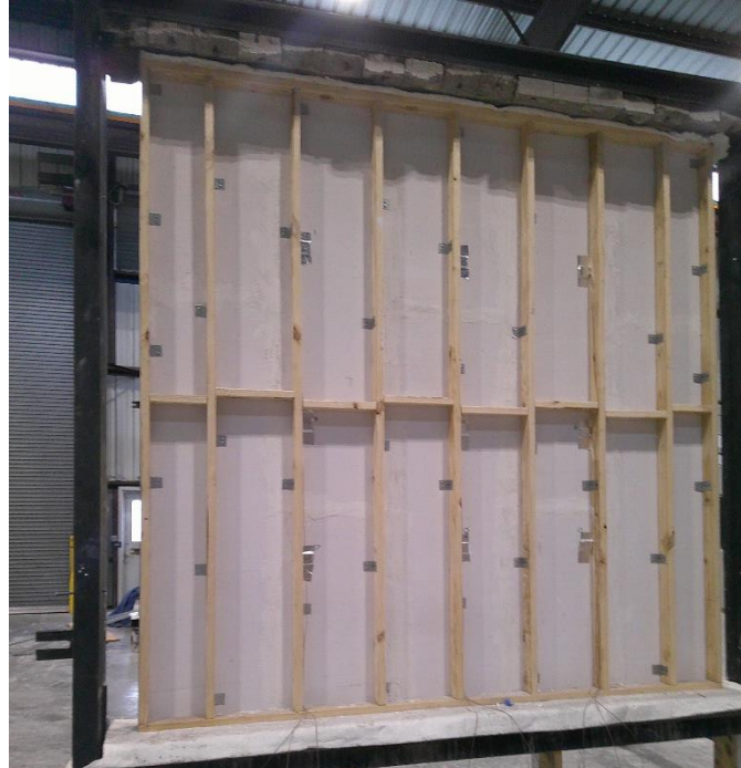
Photo No. 2 Completed installation of PAAC panels. Finish Rating Thermocouples placed on backside of panels.
