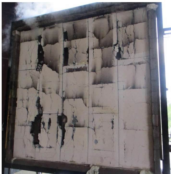
Photo No. 10 Exposed face – (Post-Hose Stream Test)
